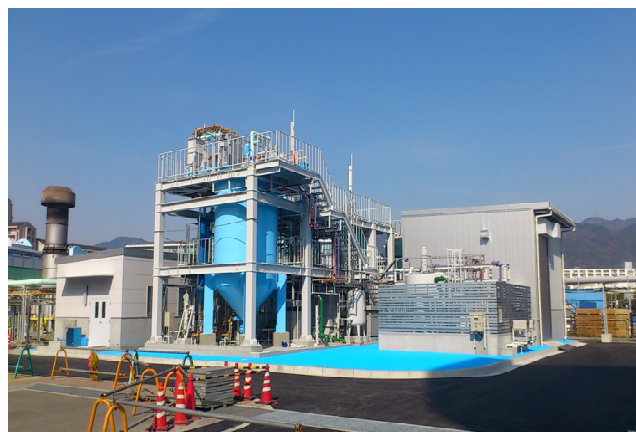
Fig. 11 Full-scale plant for recovering struvite directly from digested sludge (Higashi-Nada WWTP at Kobe). Photograph courtesy of N. Ishigami (Swing Corp.).
