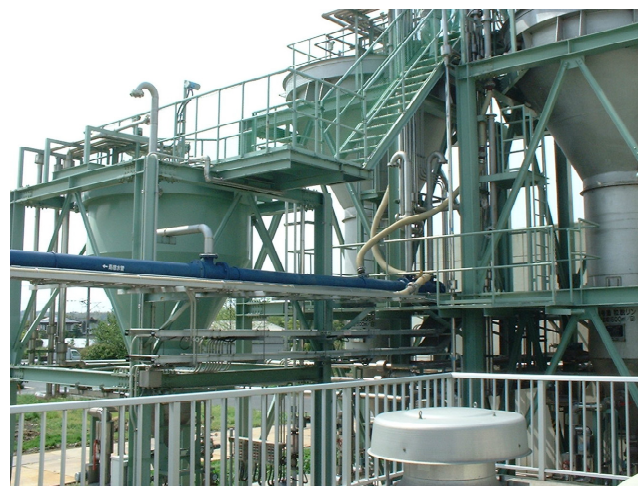
Fig. 5 Full-scale plant for recovering struvite from anaerobic sludge digestion liquor in Matsue City.
