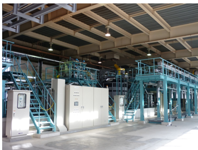
Fig. 3 Full-scale plant for recovering P from sludge incineration ash in Gifu City. Photograph courtesy of K. Goto (Gifu City Office).
